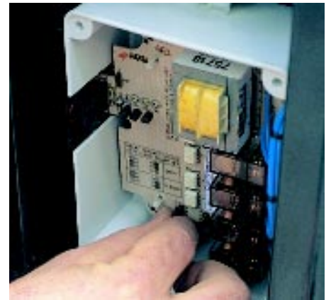
Due to size restraints inside each tower, four channel relay units were customised.
